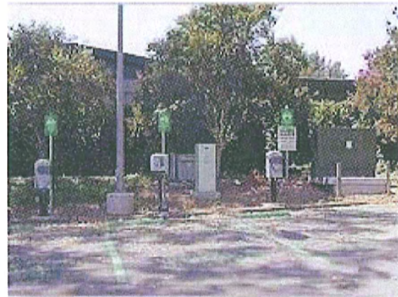
A typical Level 2 pedestal-style charging station in a surface parking lot. Photo courtesy of ECOtality.
