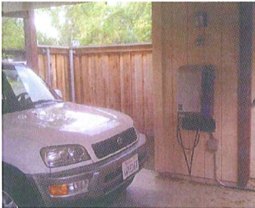
A wall-mounted Level 2 home charging station in a carport. Outdoor home charging stations can also be Level 1 and may not have to be covered. Photo courtesy of Plug In America.
