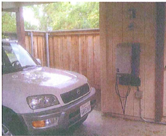
A wall-mounted Level 2 home charging station in a carport. Outdoor home charging stations can also be Level 1 and may not have to be covered. Photo courtesy of Plug In America.
