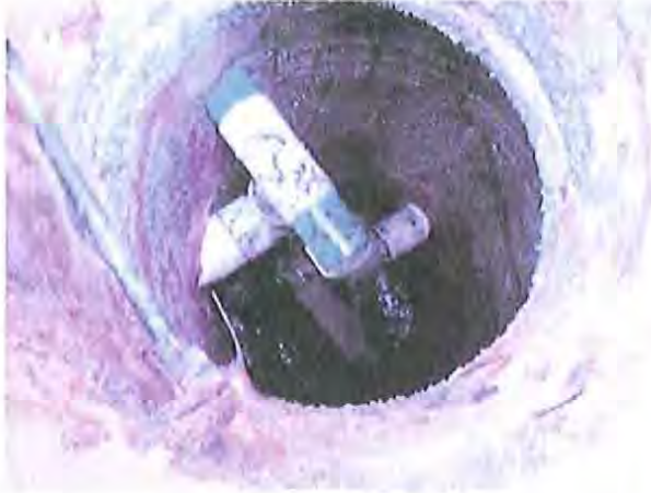
Figure 1. View Looking Down Into Manhole 4-93 Note combined PVC force main drop structure inside manhole. Exposed rebar is visible.
