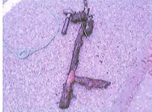
Figure 2. Corroded Neoprene Coated Access Ladder Frame Piece Removed From Manhole 4-93
