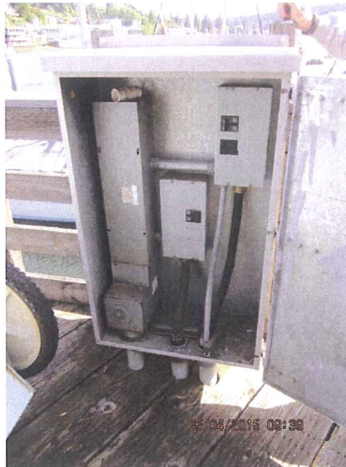
Circuit Breaker Disconnects
