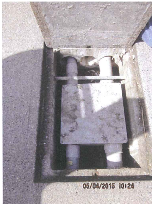
Electrical Conduit / Junction Box in Float Chase
